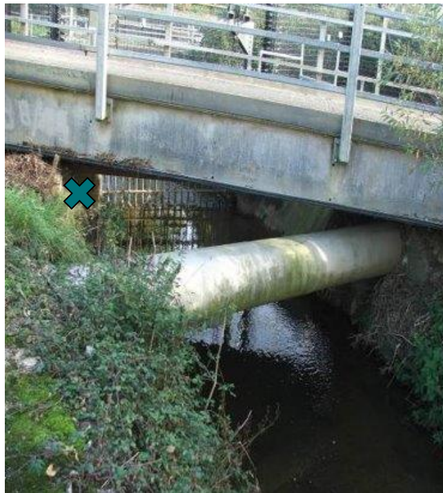
❌ Previous point of discharge into Brook
