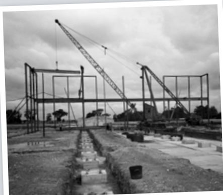
1950 Construction work began on factory-scale facilities for radioactive materials handling at the new Ministry of Supply Establishment at Aldermaston 70 years ago. Here, workers erect the steel frame for the building in which, two years later, the plutonium core will be produced for Britain's first atomic test device
